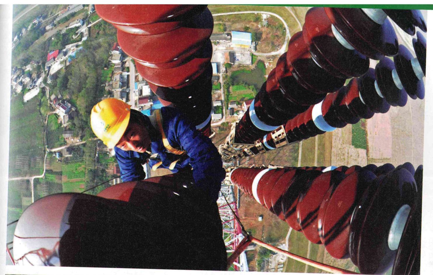
▲ Equally dangerous work is done far above the ground. This worker services an electricity pylon in the Angui province of China.
